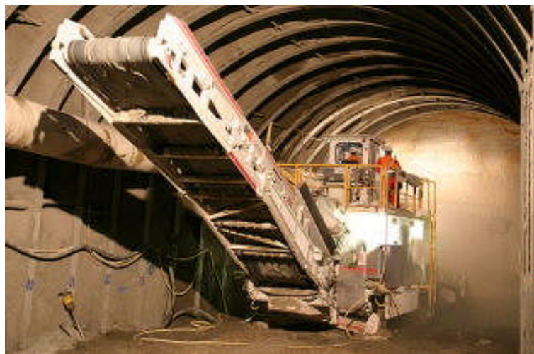
Fig 17: Lane Cove Tunnel, Sydney - Roadheader in Operation (photo courtesy of Australian Tunnelling Society).
