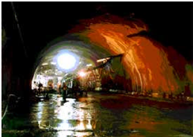
Fig 19: EastLink Tunnel, Melbourne (photo courtesy of Australian Tunnelling Society).
