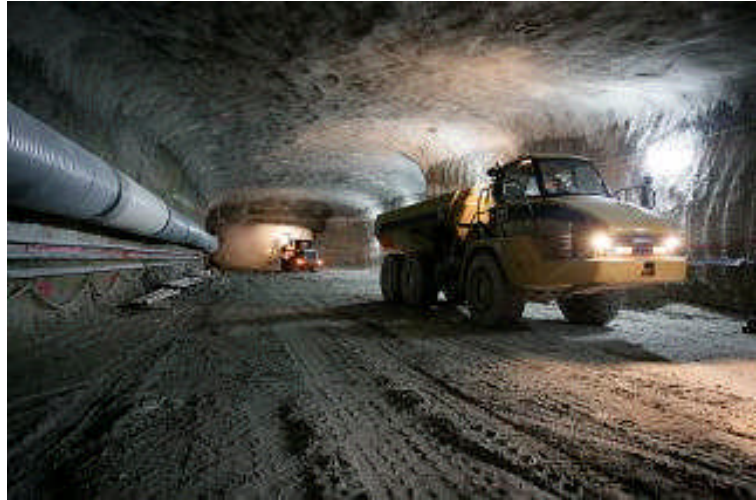
Fig 18: Lane Cove Tunnel, Sydney - Waste Removal, Ventilation Ducting and Services (photo courtesy of Australian Tunnelling Society)
