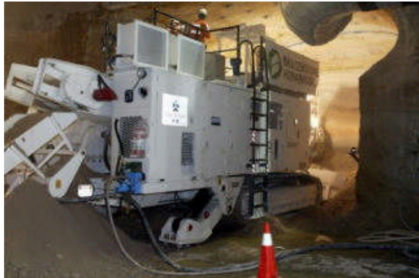
Fig 23: Cross City Tunnel, Sydney - Roadheader in Operation (photo courtesy of Australian Tunnelling Society)
